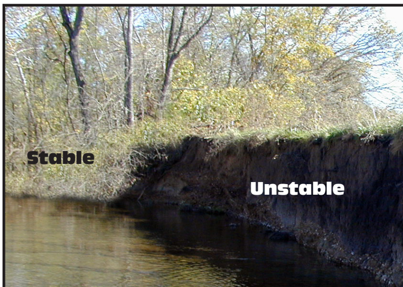
Figure 6.144 Example of stable and unstable streambank. Source: MDC
