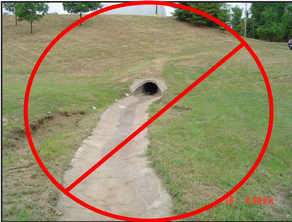
Figure 6.122 Detention basin with concrete conveyance channel. Source: Metropolitan St. Louis Sewer District
