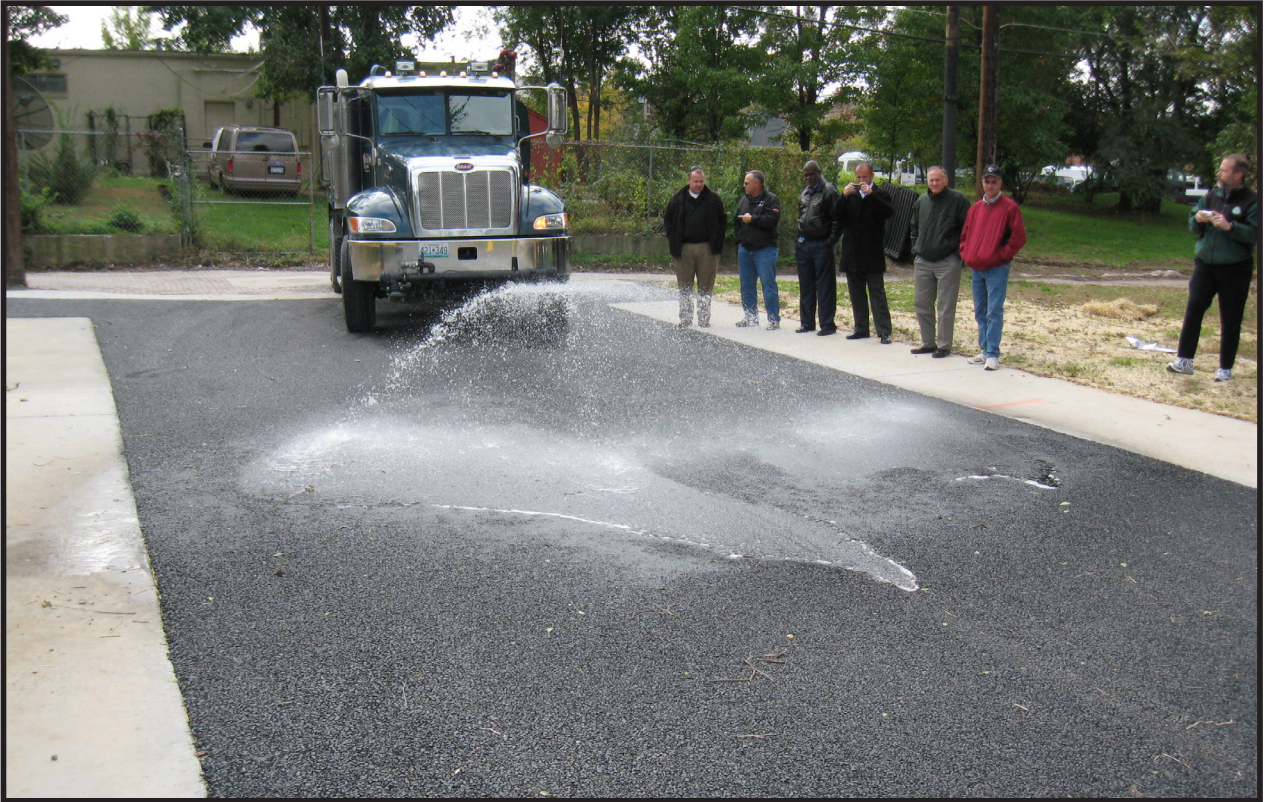
Figure 6.133: Porous Asphalt Alley, St. Louis, MO. Source: Metropolitan St. Louis Sewer District
